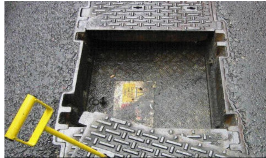
Fig 1: AboveNet chambers secured with anti-terrorist lockable lids
